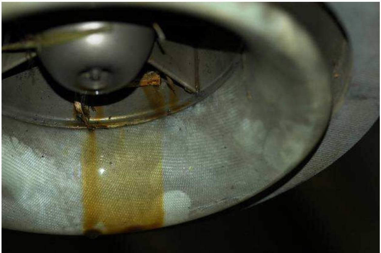
Figure 21. Traces of oil leakage
